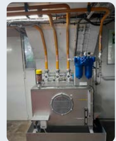
Centrale lubrification Paliers
