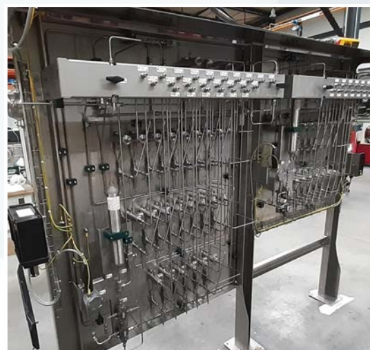
Control PANELS ATEX
